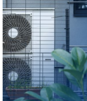
HEAT PUMPS COMPONENTS
